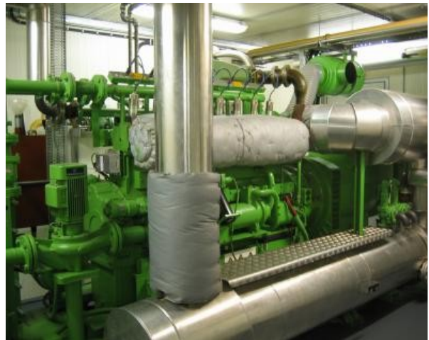
The installation of a CHP system dramatically reduces energy costs
